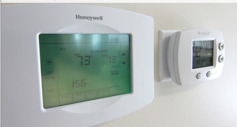
New temperature-control system.
